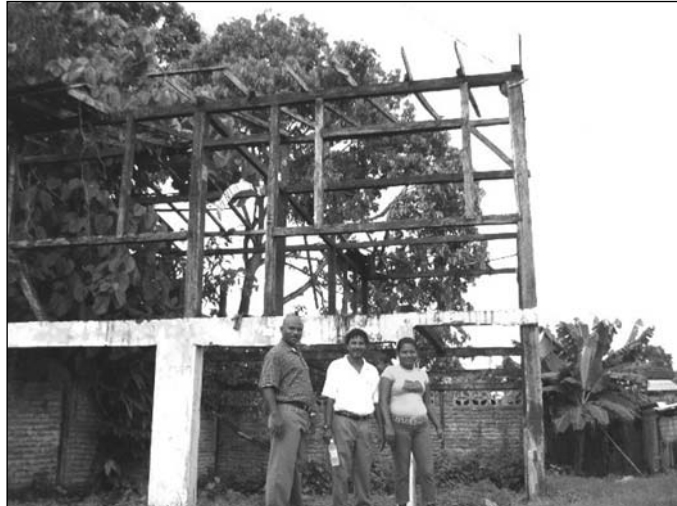
Members of the local action committee in Esmeraldas, Ecuador. A large number of buildings in the town were damaged by a fire caused by an extensive oil spill
